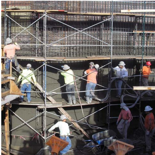
Shooting concrete on the wall of the ramp between the Basement and First Level parking
