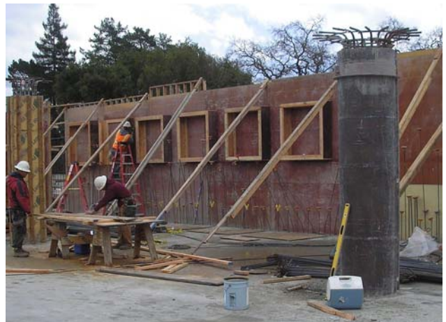
Looking at the south wall of the First Level parking – the squares will be openings beneath the Children’s Activity Deck on the Second Level
