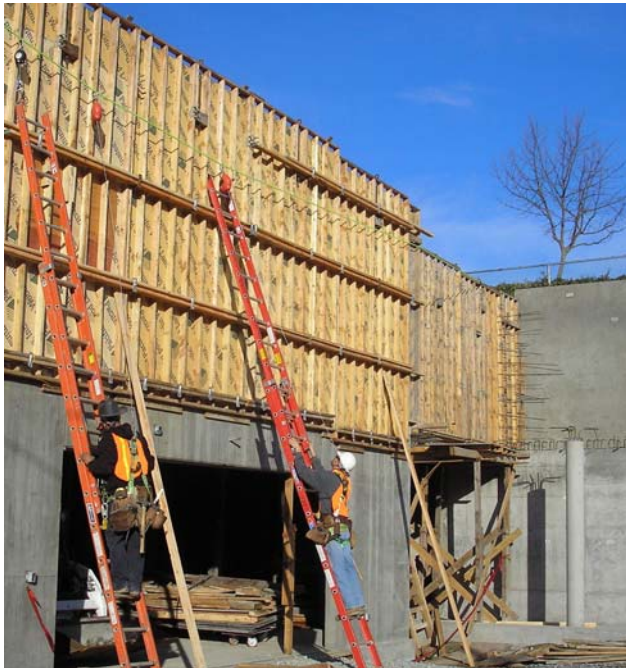
Preparing the First Level wall above the Parking Garage entrance -- Column for solar panel at right of photo
