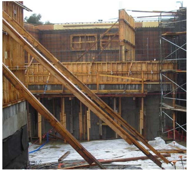
Looking at the wall of the Bicycle Room and Emergency Generator Room from the ramp between parking levels
