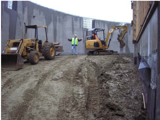
The parking ramp between the Basement and First Level parking areas – January 11th
