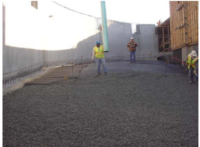
The parking ramp between the Basement and First Level parking areas – January 15th
