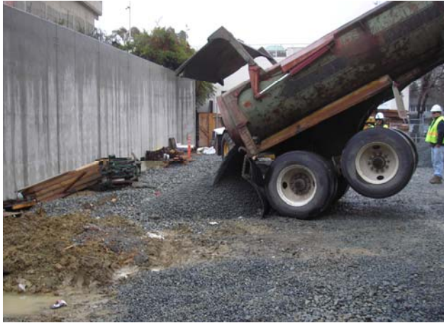
#1 – Gravel is unloaded in the parking lot in front of the shoring wall below Boswells.
