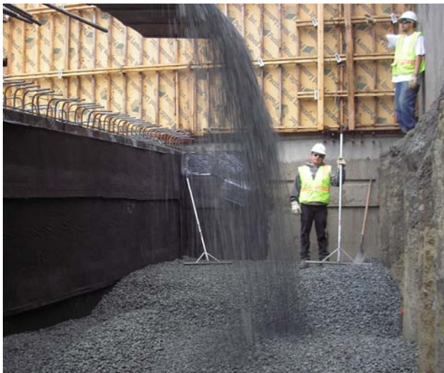
#3 – Gravel is poured into the space between the shoring wall and Boswell's retaining wall.
