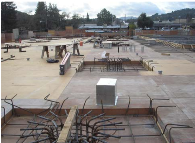
Looking west at decking on the Second Level over the rebar and conduit
