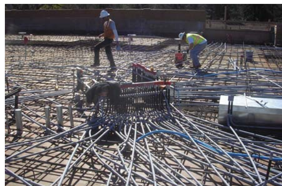
Cabling and conduits on Second Level
