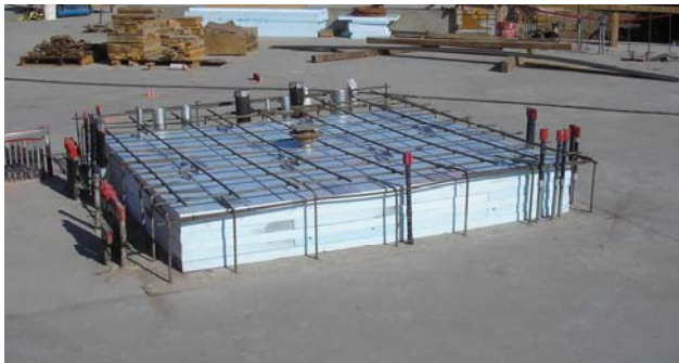
Utility connections in Children's Area's Family Restroom
