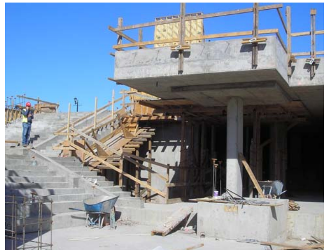
Looking up Plaza Staircase and Teen Area (cantilevered section) from the Reading Plaza
