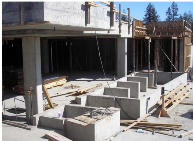
Planter and shade fin supports in the Reading Plaza in front of Arts & Science Discovery Center
