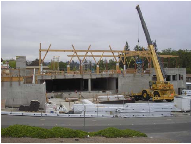
Installation of heavy timber system on the second deck over the Arts & Science Discovery Center
