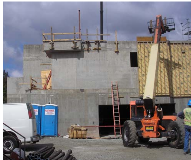
Looking west at the Parking Garage entrance – the overhang at the top left is the Storytelling Corner in the Children’s Area
