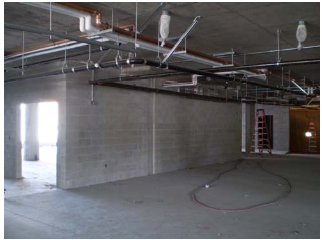
Utility lines along parking garage ceiling
