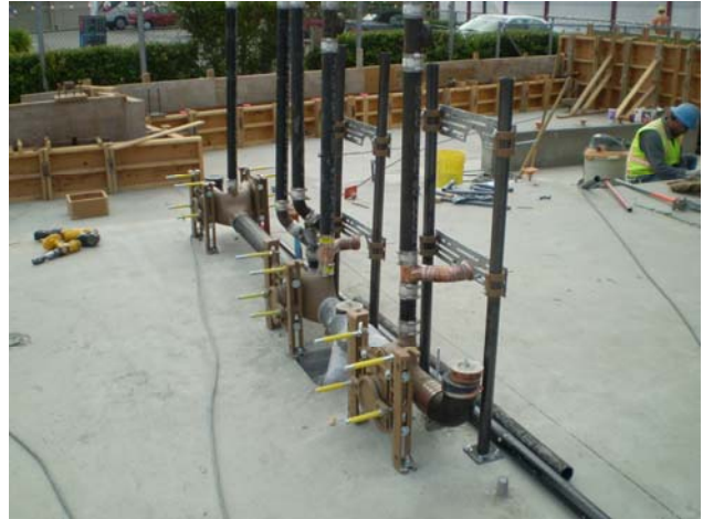
Plumbing connections for the public restrooms off the Entrance & Lobby
