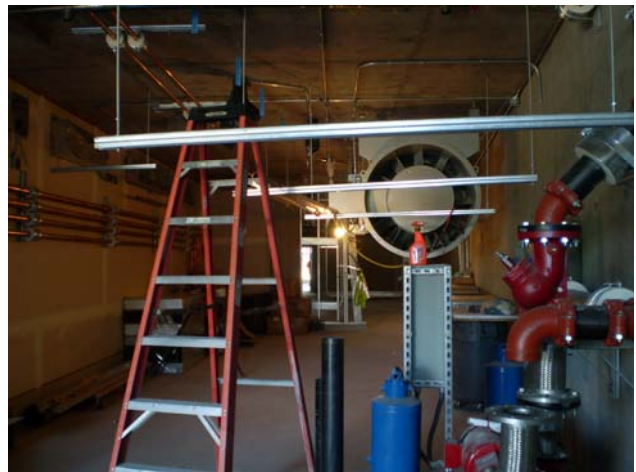
First Level Mechanical Room
