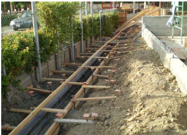
Footing for wall on the eastern property line Seaborg Garden is at the right
