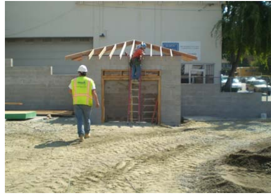
Trash enclosure at the east end of the parking lot
