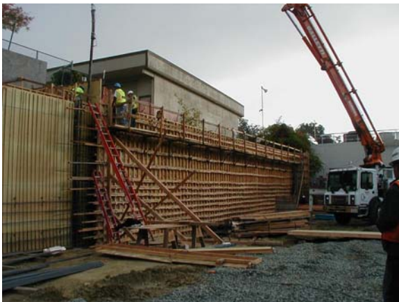
Formwork for the retaining wall in the Parking Lot below Boswells was completed, and concrete was pumped into forms
