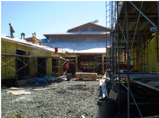
Looking south into the Main Plaza to the Library Entrance & Lobby with weatherproofing on Staff Wing roof at the right
