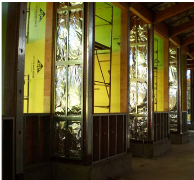
Insulation around the Family Reading nooks in the Children's Area
